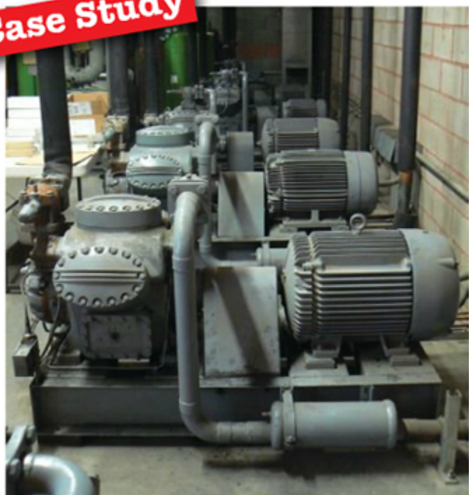
These Carrier open-drive reciprocating compressors were part of the Food 4 Less supermarket's refrigeration system that was converted from R-22 to R-407F by RSI of West Sacramento. (Photo by Ted Rieger)
